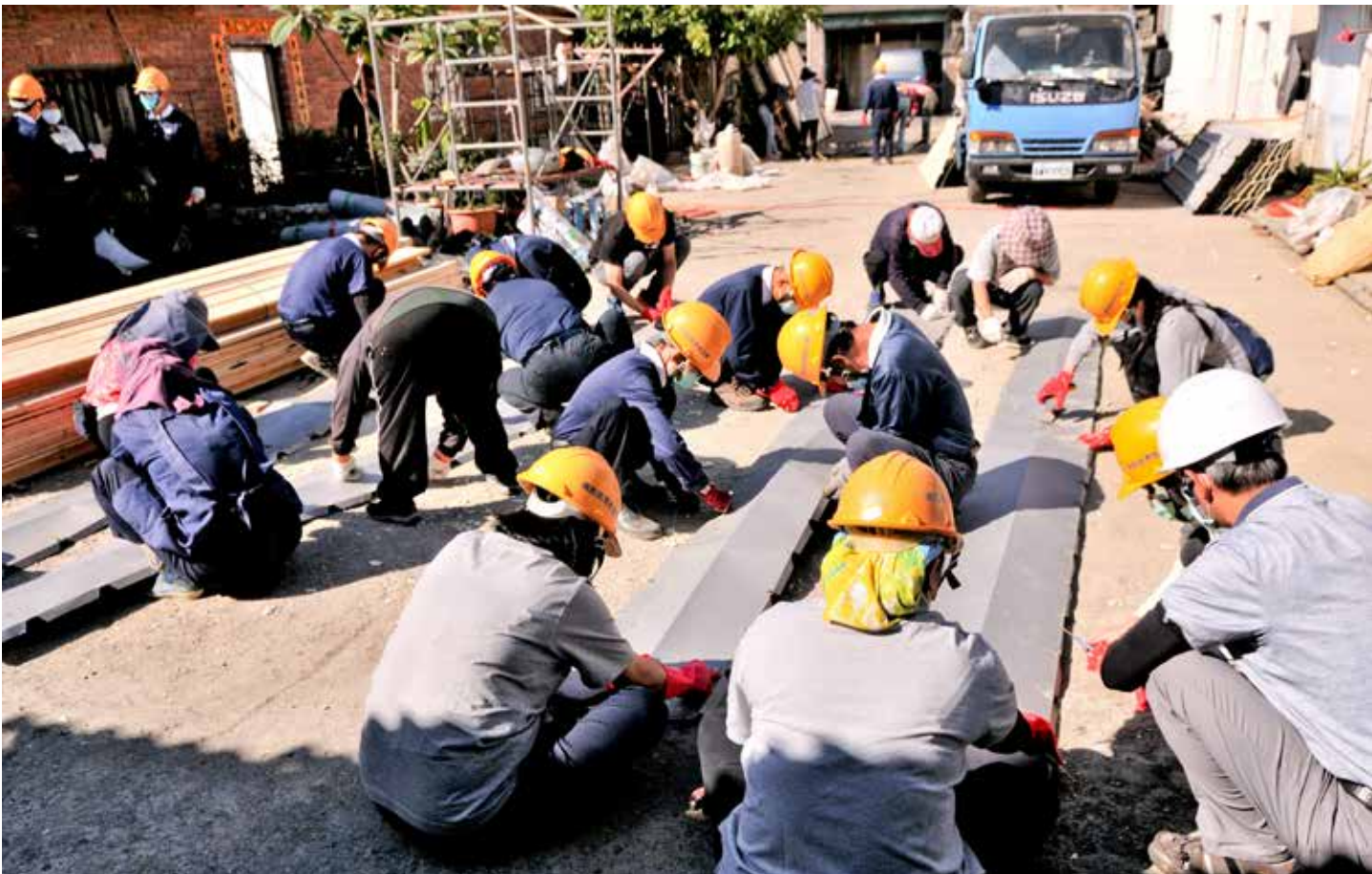
Douliu Tzu Chi Hospital cooperated with the Tzu Chi Foundation Construction Office and Yunlin Tzu Chi volunteers to repair houses for care recipients.
