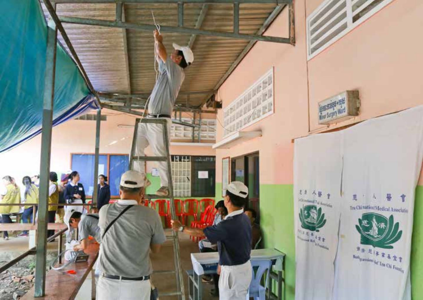
The hallway of the free clinic has poor lighting system. Volunteers work diligently to install the lights.
